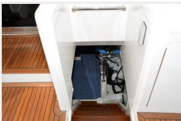
Walk-in Engine Room Access
