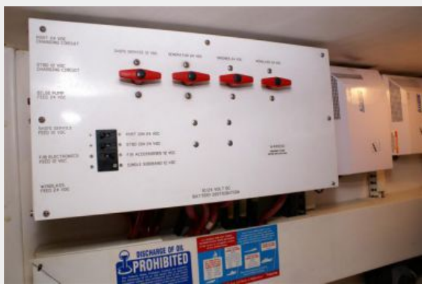
Battery Distribution Panel
