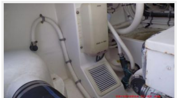
Engine & Mechanical Equipment 7
