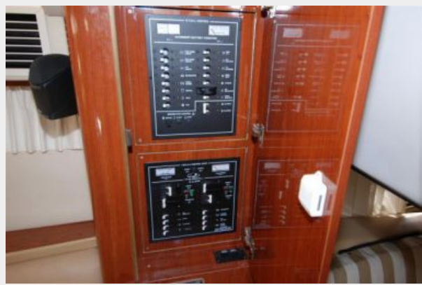
Power Panel in Salon
