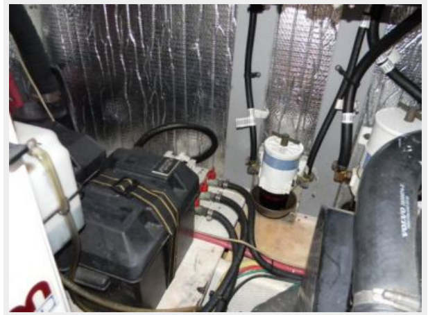
STBD Engine Room
