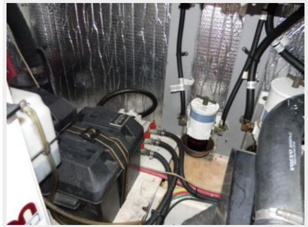
STBD Engine Room
