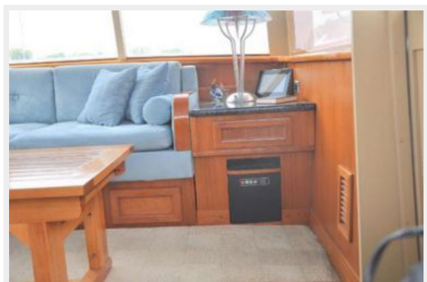
AC Heater hard wired
