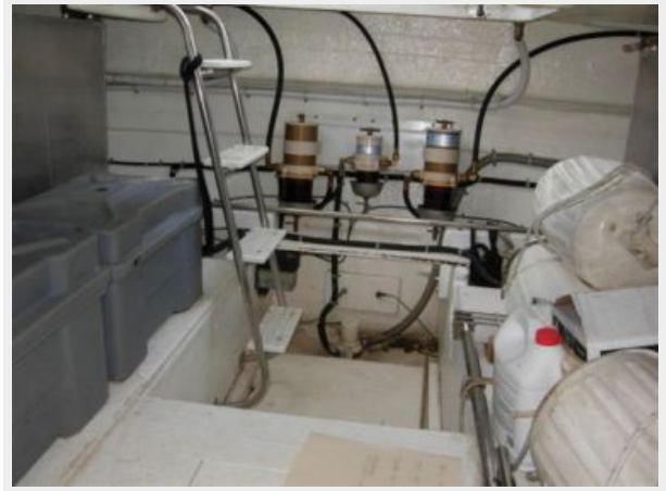
engine room fwd
