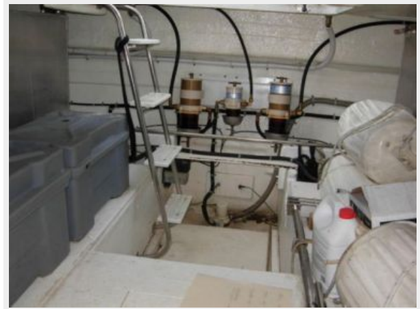
engine room fwd
