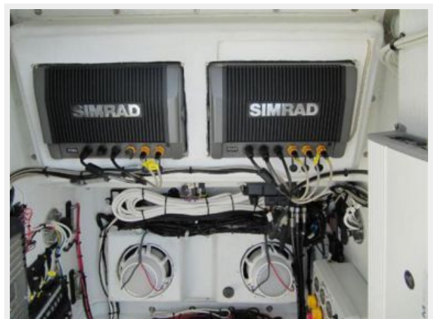
Under Helm Electronics
