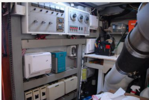
Engine Room / Aft Port
