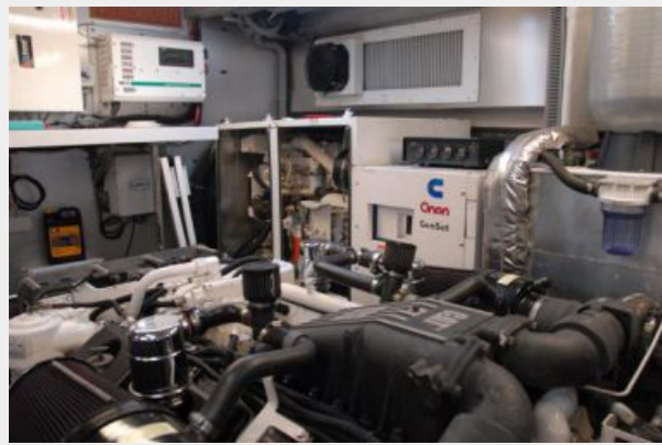
Engine Room / Forward to Starboard
