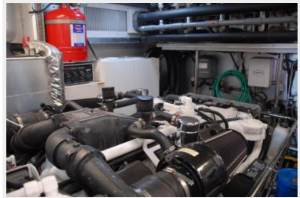
Engine Room / Forward to Port
