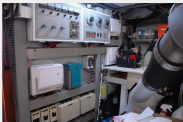
Engine Room / Aft Port
