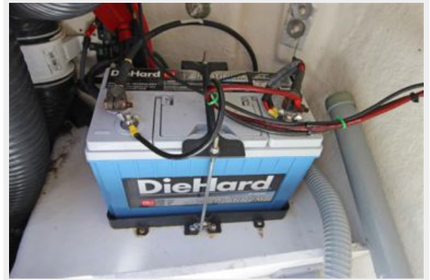
Battery Mounted In Tray
