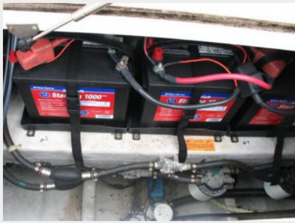
Electrical System / Equipment - Batteries
