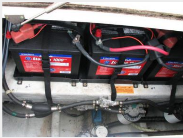
Electrical System / Equipment - Batteries
