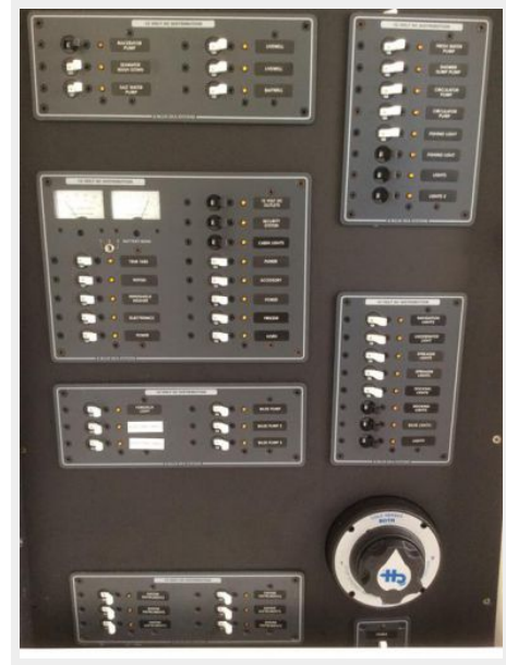
Power panel inside console
