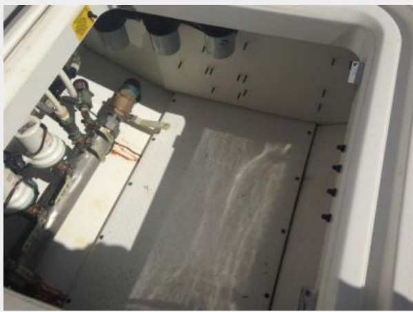
Bilge, fuel water separators
