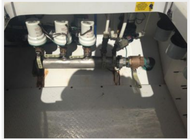
Bilge, livewell pumps with manifold
