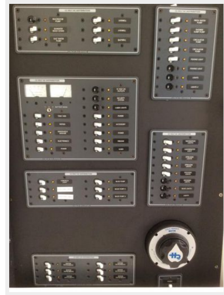
Power panel inside console
