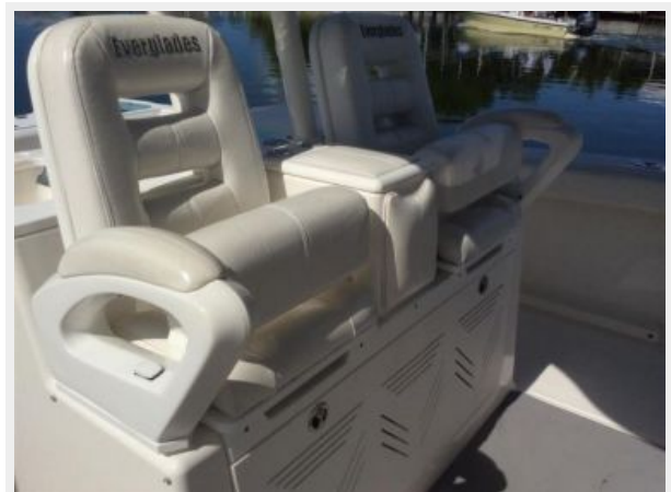
Battery compartment below helm seating
