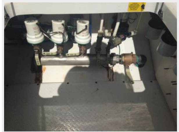
Bilge, livewell pumps with manifold
