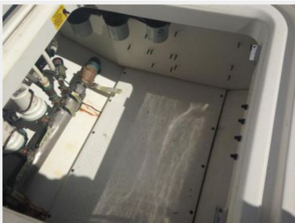
Bilge, fuel water separators
