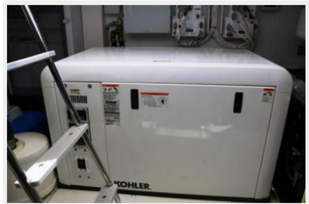
Engine Room Generator
