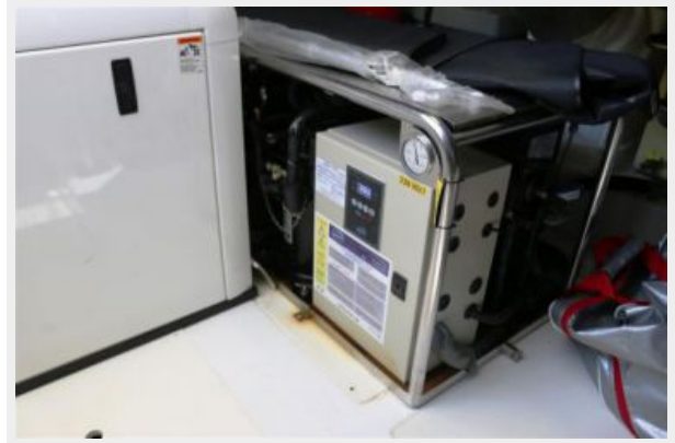
Engine Room AC Chiller
