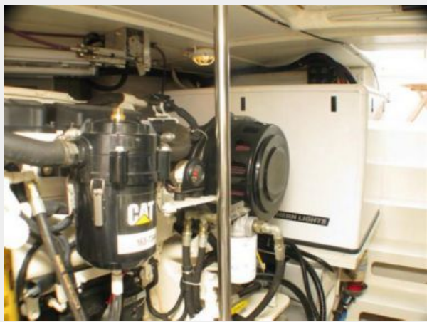
Stern Lights Generator With Enclosure
