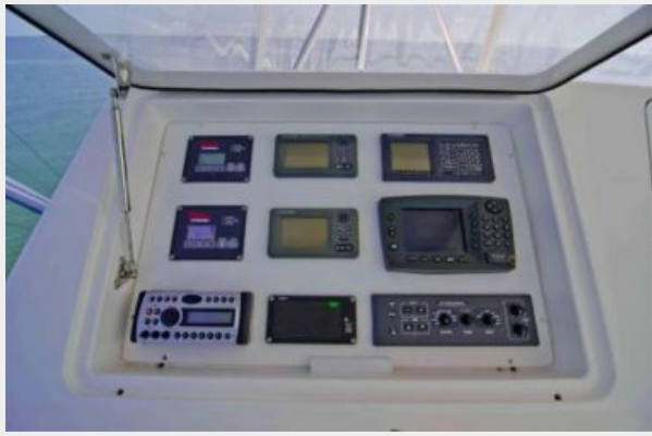
Flybridge Helm Electronics
