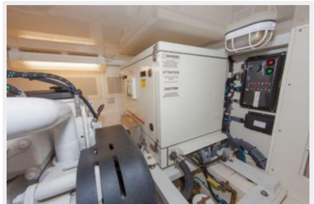
Engine Room Port Forward with Generator
