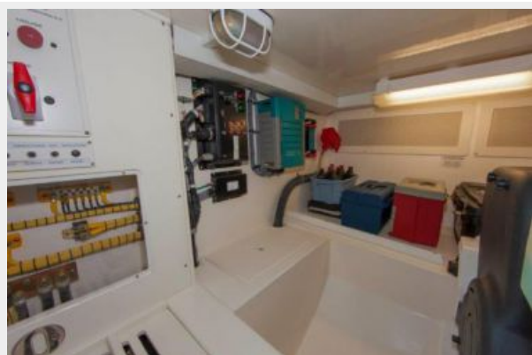
Engine Room Starboard Forward
