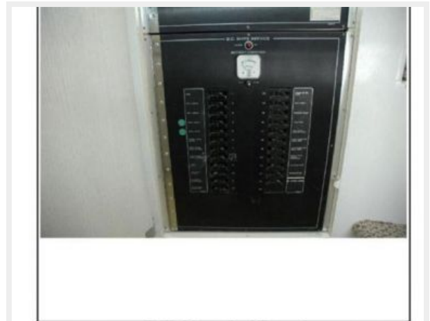
DC Electrical Panel
