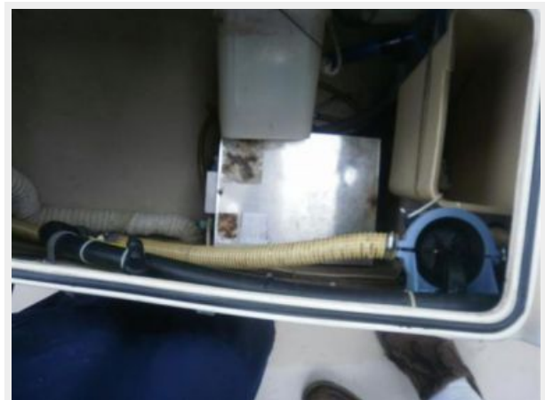
6-Gallon Hot Water Heater
