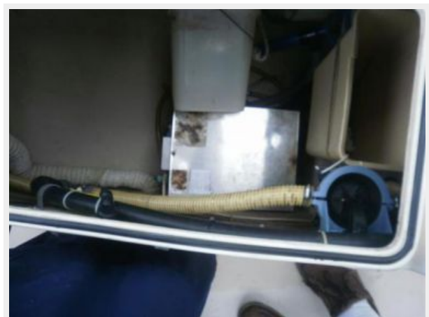
6-Gallon Hot Water Heater
