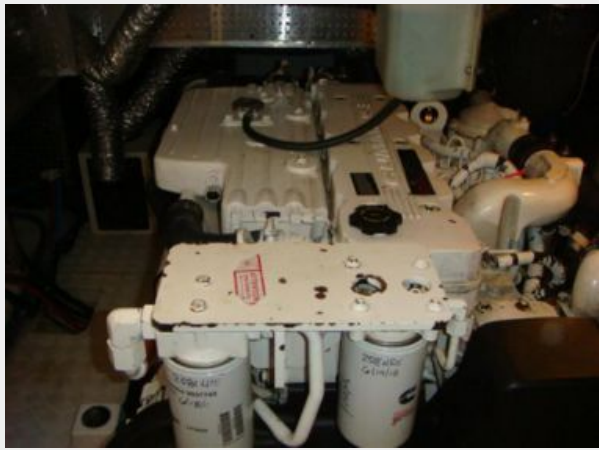
37' Mariner Seville engine room aft
