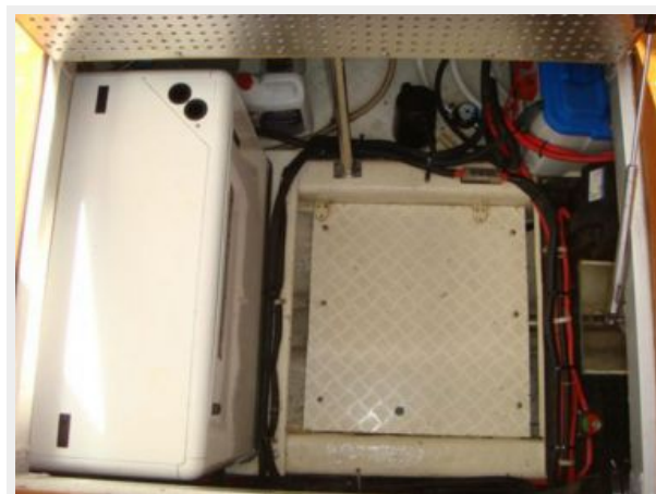
37' Mariner Seville engine room aft access
