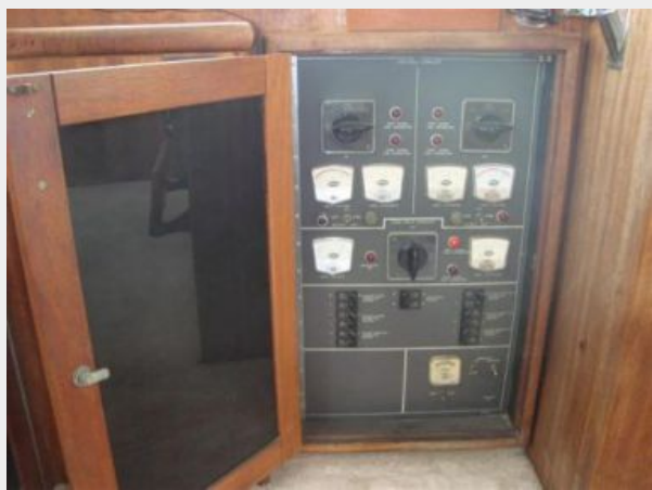
AC breaker panel
