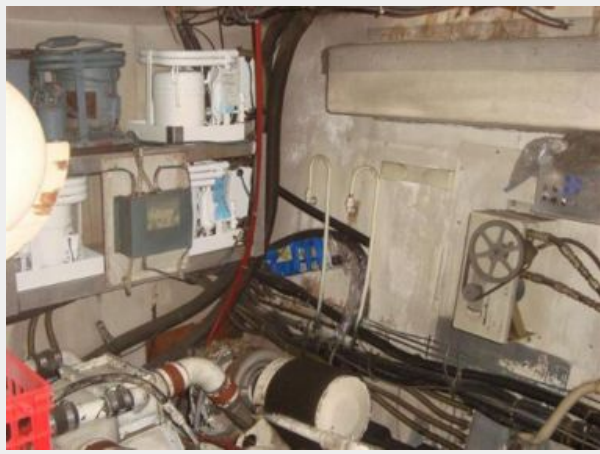
Port engine room
