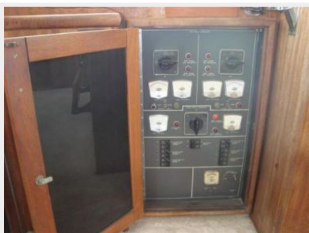
AC breaker panel
