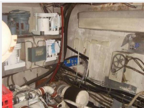
Port engine room
