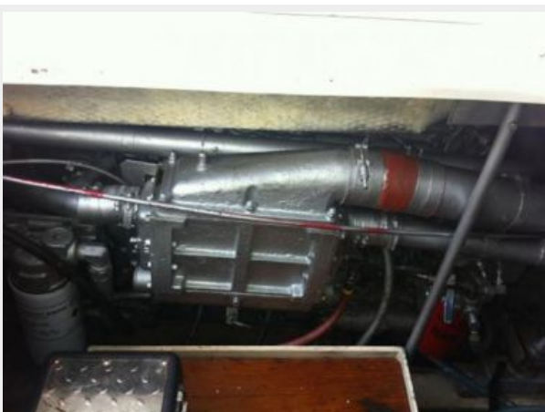
Engine room (strb)
