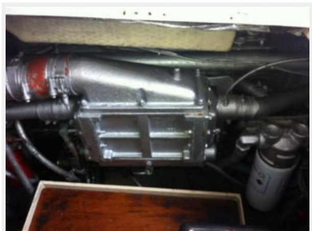
Engine room (port)
