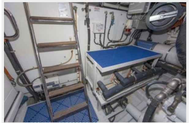
Chilled Water AC
