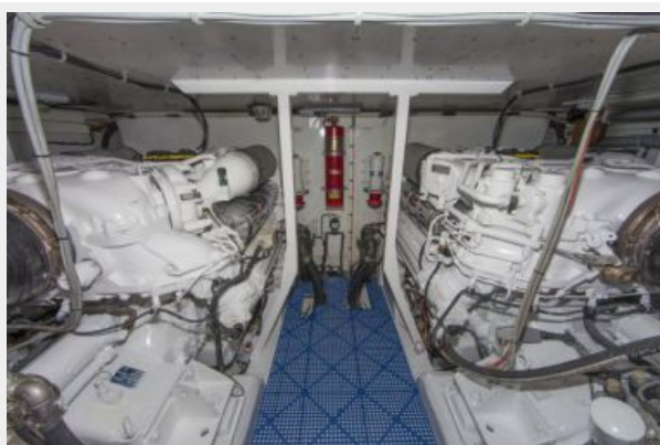
Engine Room Looking Forward
