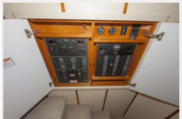
Companionway Electrical Panel
