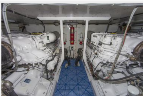
Engine Room Looking Forward
