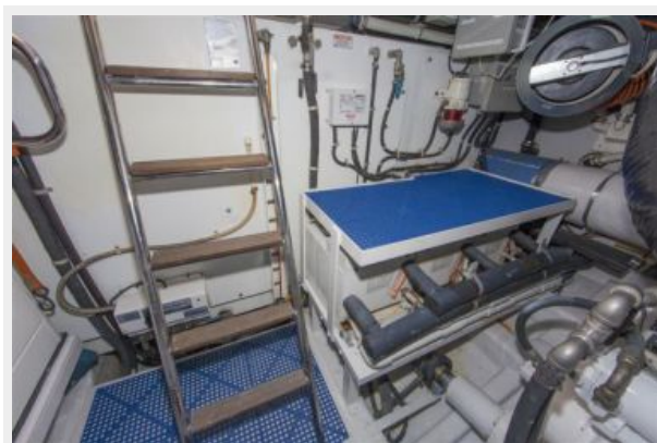
Chilled Water AC
