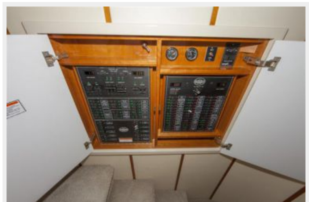
Companionway Electrical Panel
