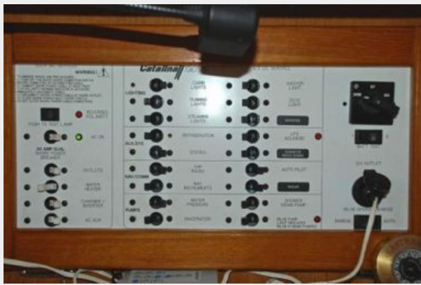
Main Breaker Panel
