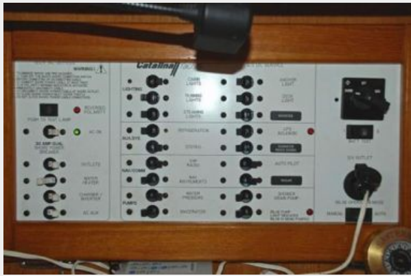
Main Breaker Panel
