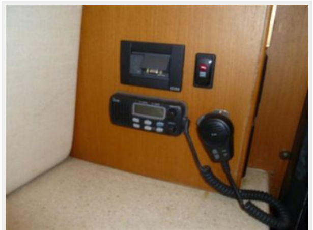
Salon backup VHF
