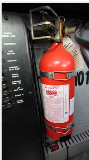
Engine Room Fire Suppression
