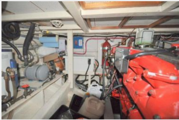
Engine Room Detail
