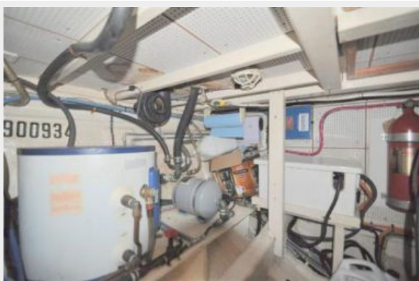
Engine Room Detail
