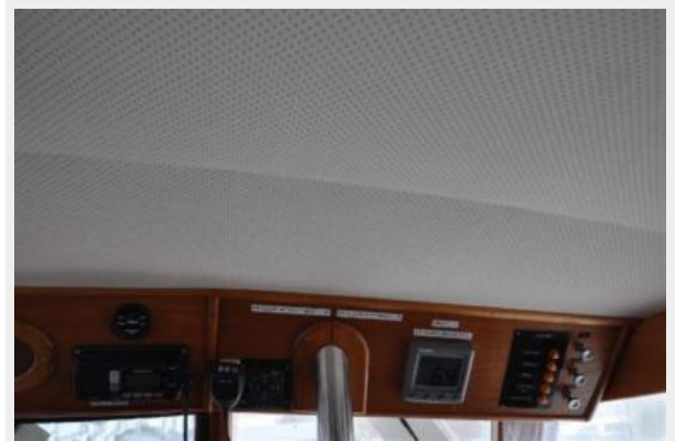
wheelhouse overhead electronics
