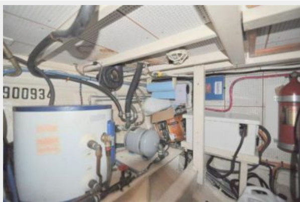
Engine Room Detail
