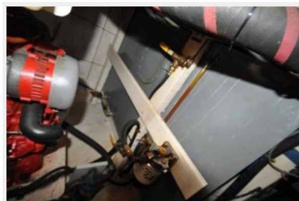
Engine Room Detail
