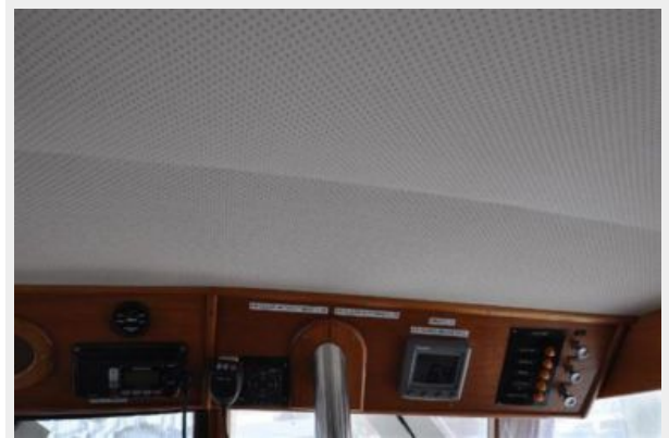
wheelhouse overhead electronics
