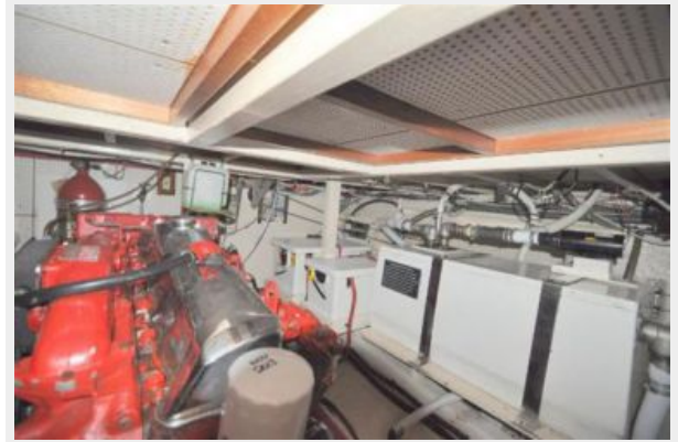
Engine Room Detail
