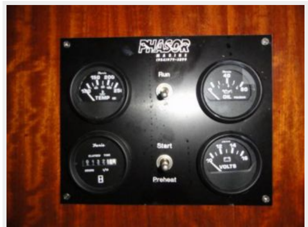
Salon Generator Control
