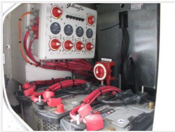
Electrical System / Equipment
