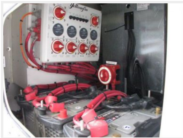
Electrical System / Equipment
