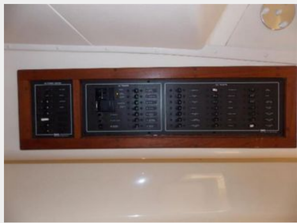
'02 Carolina Classic 35, AC/DC breaker panel and remote generator controls
