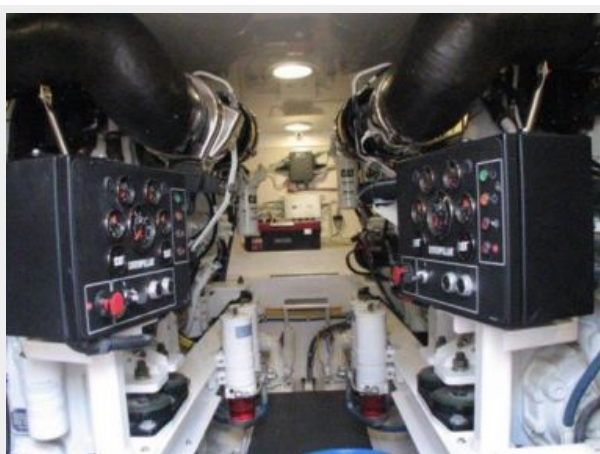
Engine & Mechanical Equipment 1 - Engine Room
