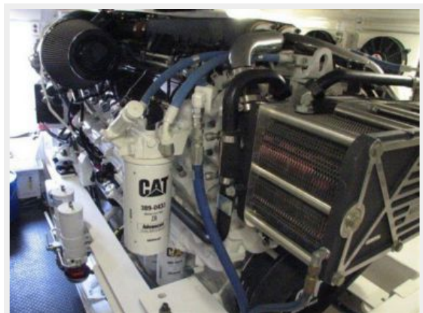
Engine & Mechanical Equipment 2 - Port Engine
