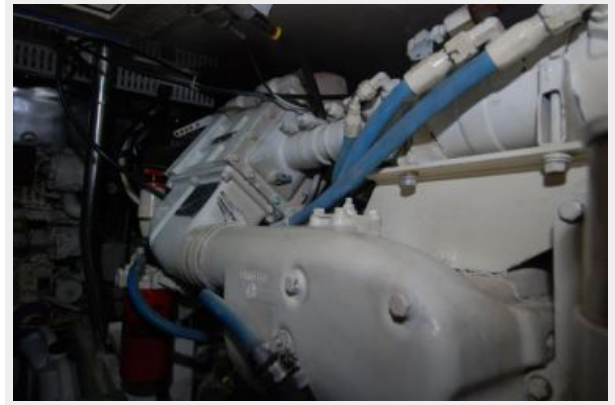
Engine Room facing aft
