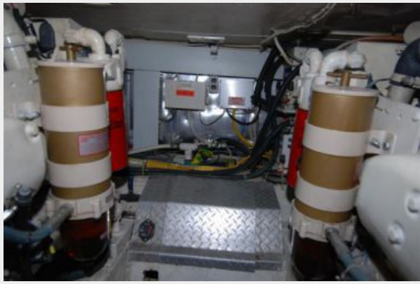
Engine Room looking forward
