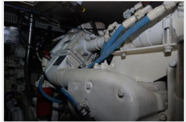
Engine Room facing aft
