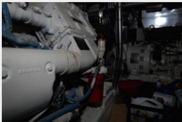
Engine Room facing aft
