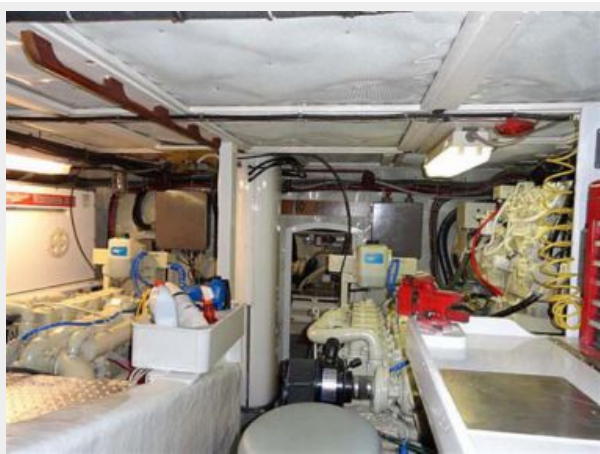
Engine Room, Looking Forward
