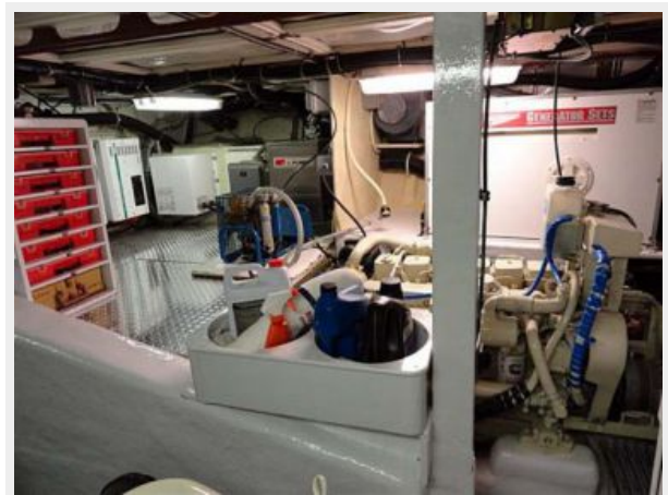
Engine Room, Port
