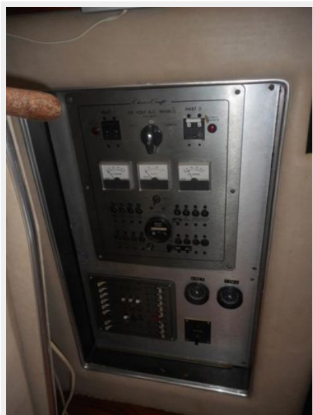
38' Chris Craft electrical panel
