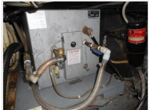
38' Chris Craft water heater
