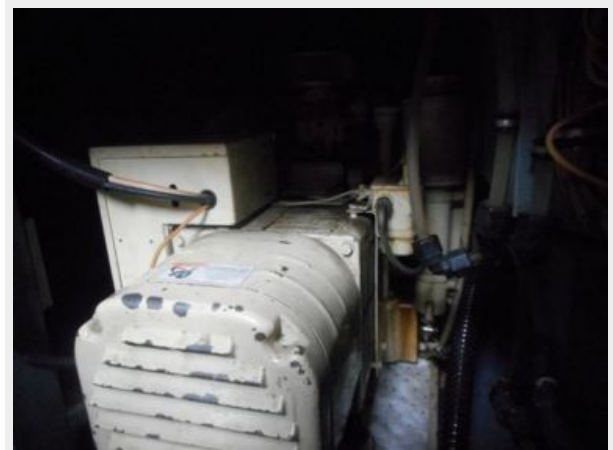
38' Chris Craft generator
