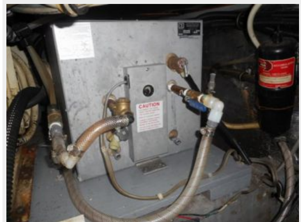
38' Chris Craft water heater
