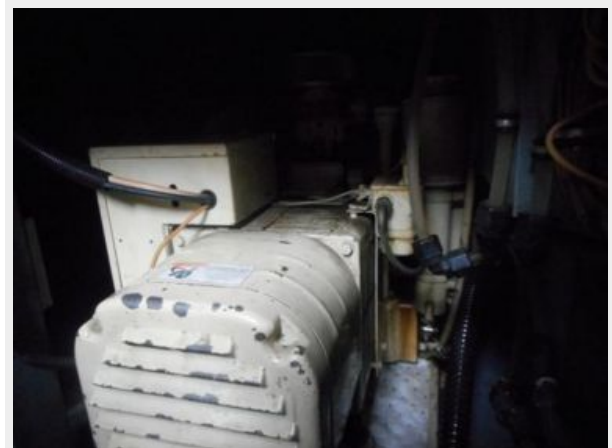
38' Chris Craft generator
