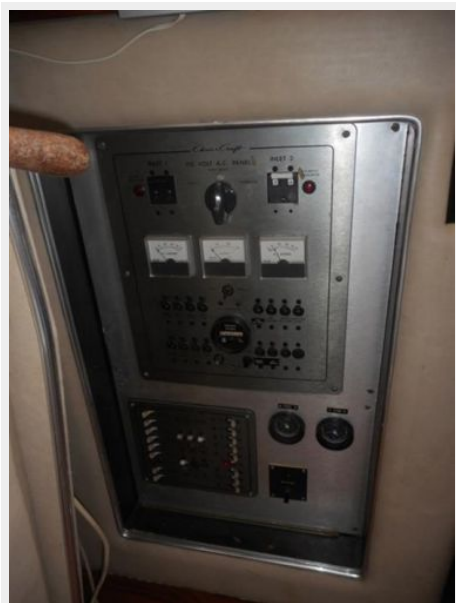
38' Chris Craft electrical panel
