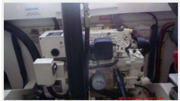
Electrical System / Equipment 3 - Generator
