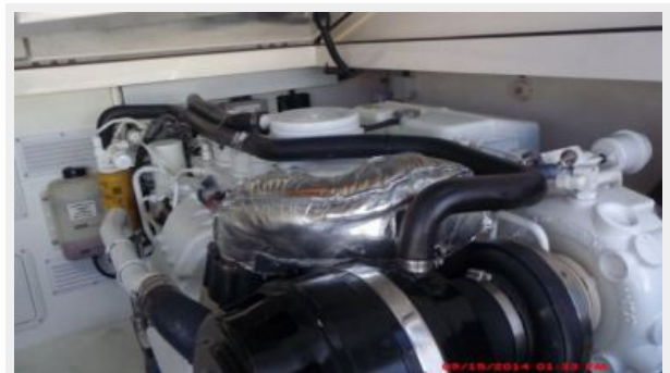
Engine & Mechanical Equipment 2
