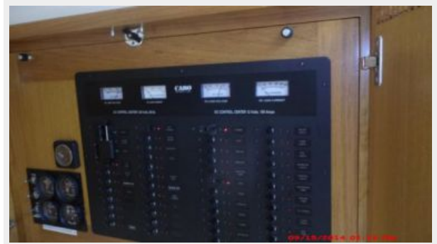
Electrical System / Equipment 1 - Electrical Panel
