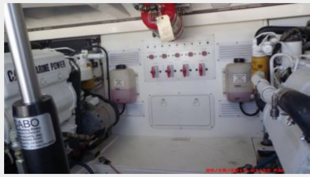
Engine & Mechanical Equipment 3
