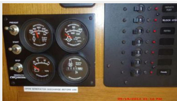
Electrical System / Equipment 2 - Electrical Panel
