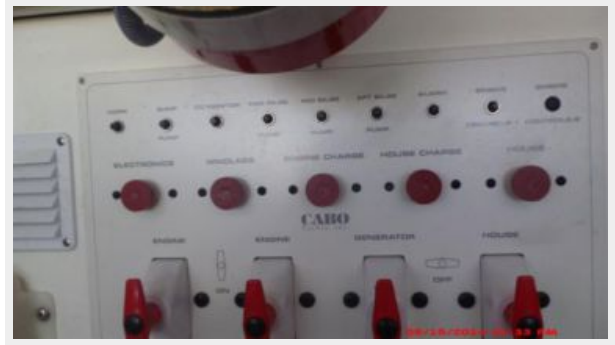
Engine & Mechanical Equipment 4
