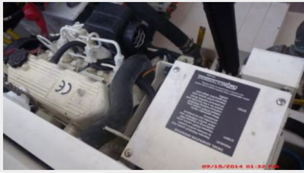
Electrical System / Equipment 4 - Generator
