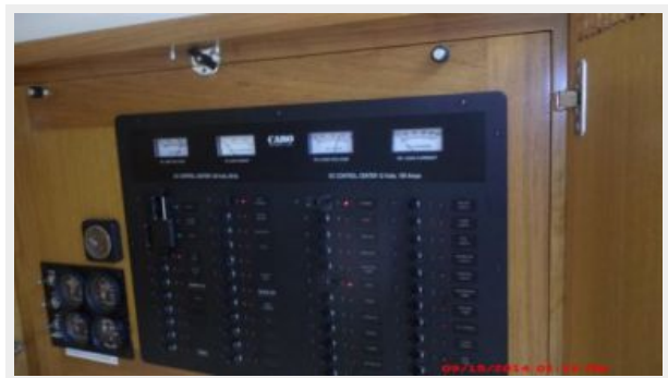
Electrical System / Equipment 1 - Electrical Panel
