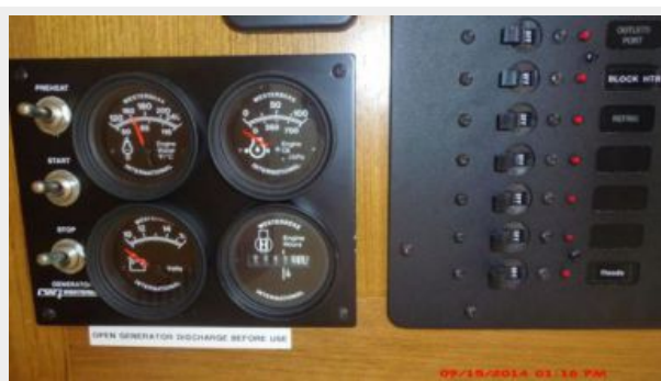
Electrical System / Equipment 2 - Electrical Panel
