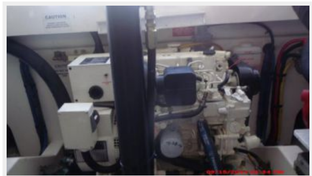
Electrical System / Equipment 3 - Generator
